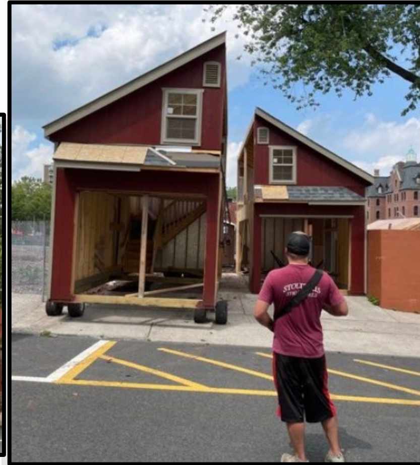
Modular garage installation. Left and right – installation in progress. Center – installation complete.
