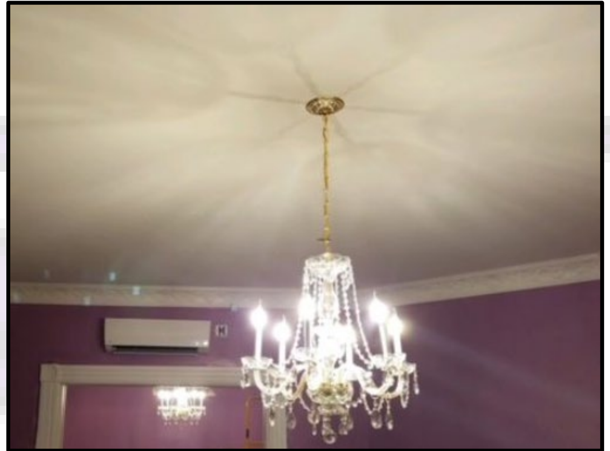
New chandeliers and lighting fixtures (Dining Room and Front Chapter Room).
